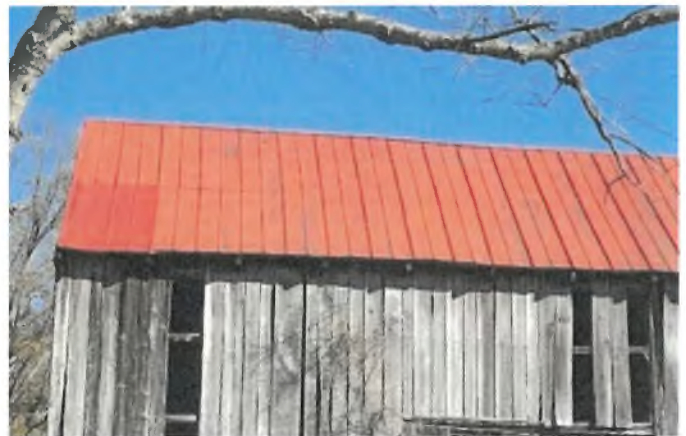
The metal roof of this tobacco barn at Cedar Hill, Prince Frederick has been patched and repaired. Image courtesy of Calvert County.
